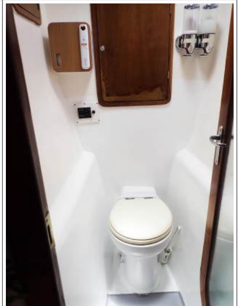
Electric toilet, forward starboard (Adventurer)
